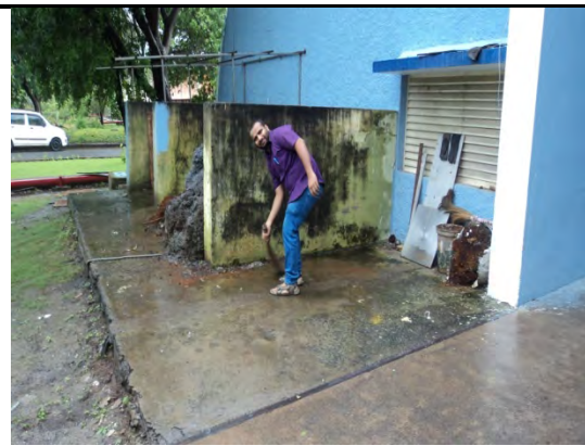
Shutter right side Before cleaning
